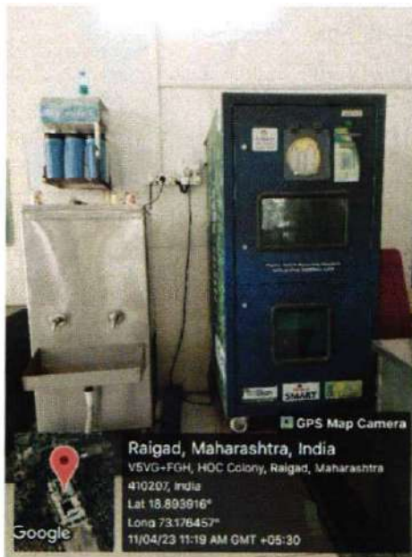
Photo: Water Cooler
