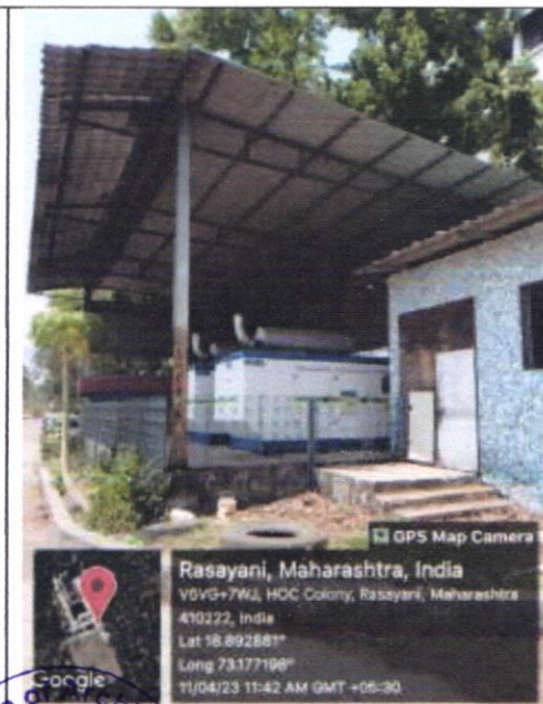
Generators for power backup
