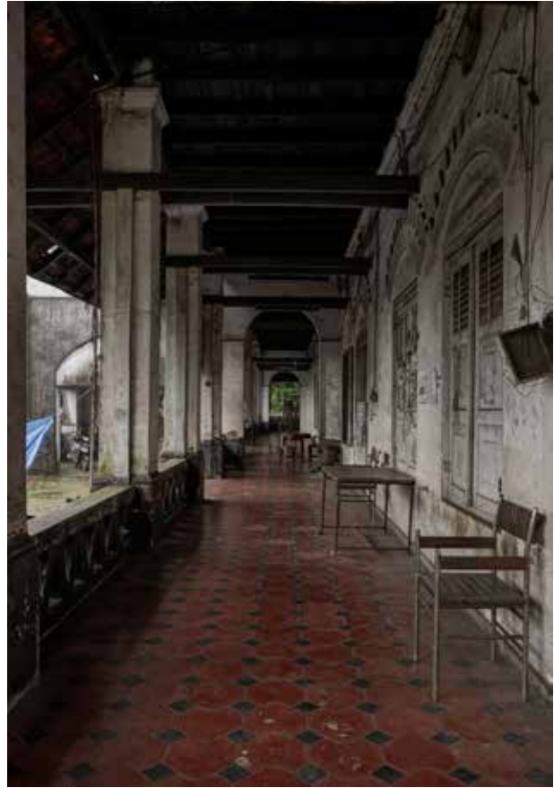
The long verandah of the main building facing the Manachira is paved with clay tiles were from the Comtrust Tile factory of Puthiyara.
