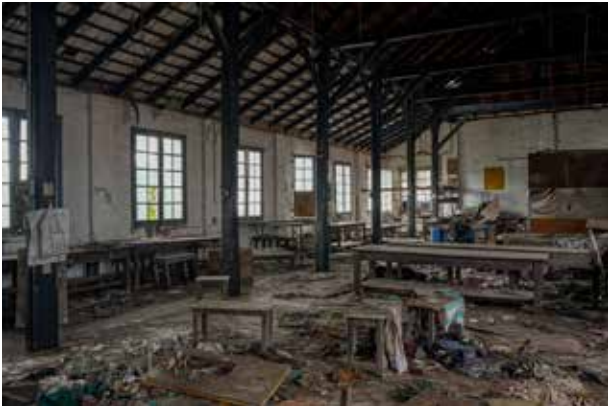
The large godown in first floor of the main building used for packing and labelling for the finished products. These large racks still have the finished products untouched, as left 20 years ago. Single piece logs are used as columns.
