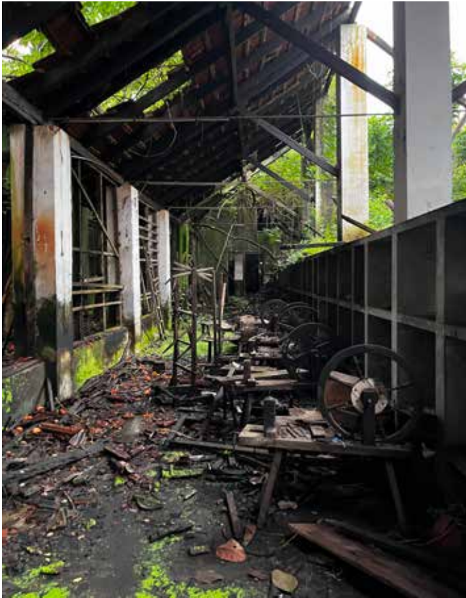
Adding to the dilapidating condition of the wooden roof supports, the recent incidents of heavy rains have caused the roofs to cave in. The charkas can be seen in a room near the looms.
