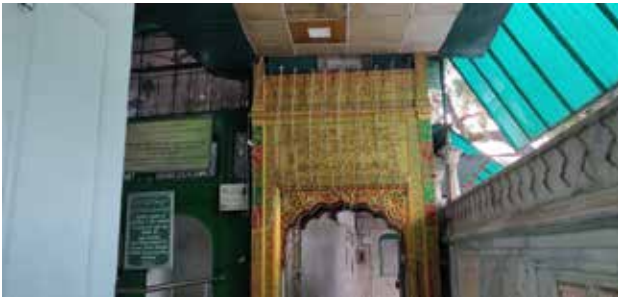
Figure 8: The state of collapse of the roofing of the Dargah. (Source: Author)
