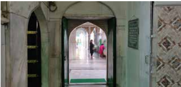
Figure 9: Tiling done on the Dargah by the committee- an insensitive intervention. (Source: Author)
