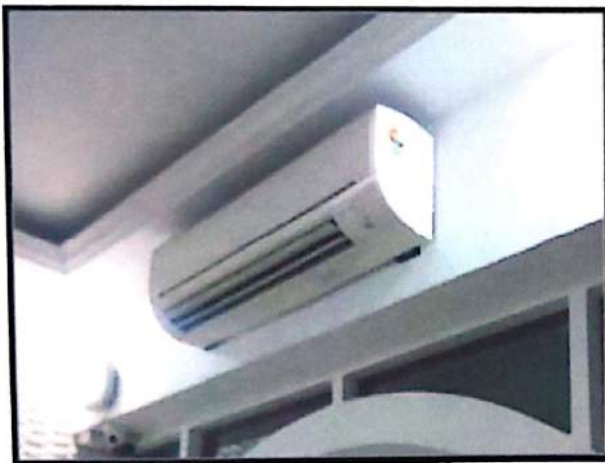
Air Conditioners Installed in Lab
