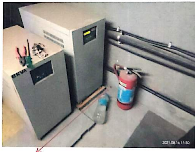
Fire extinguisher are provided but 5 ft. on wall mounted
