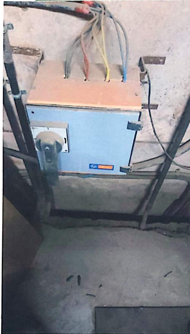
Electrical Insulating mat is provided on flooring.
