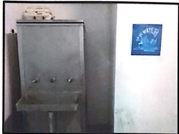
Signages near Cooler/Purifier
