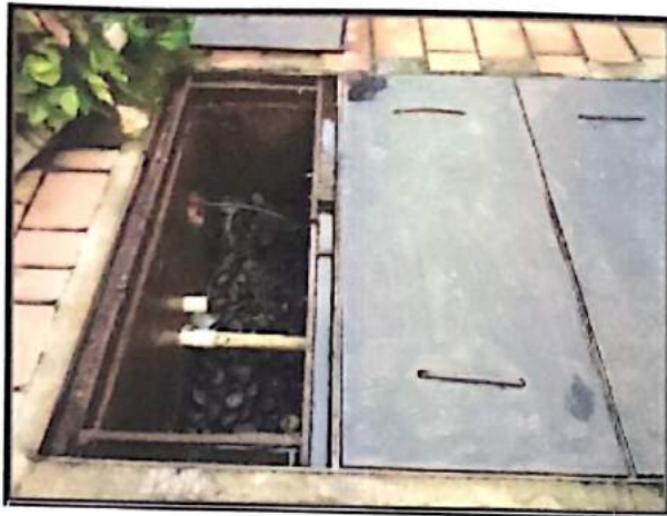
Rainwater Harvesting System- Recharge Pit
