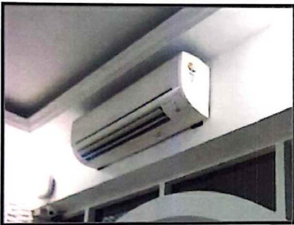
Air Conditioners Installed in Lab
