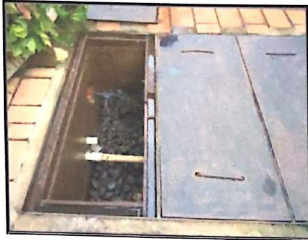
Rainwater Harvesting System- Recharge Pit
