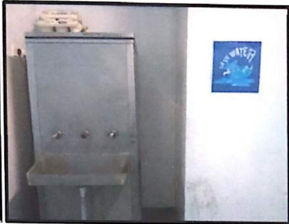
Signages near Cooler/Purifier
